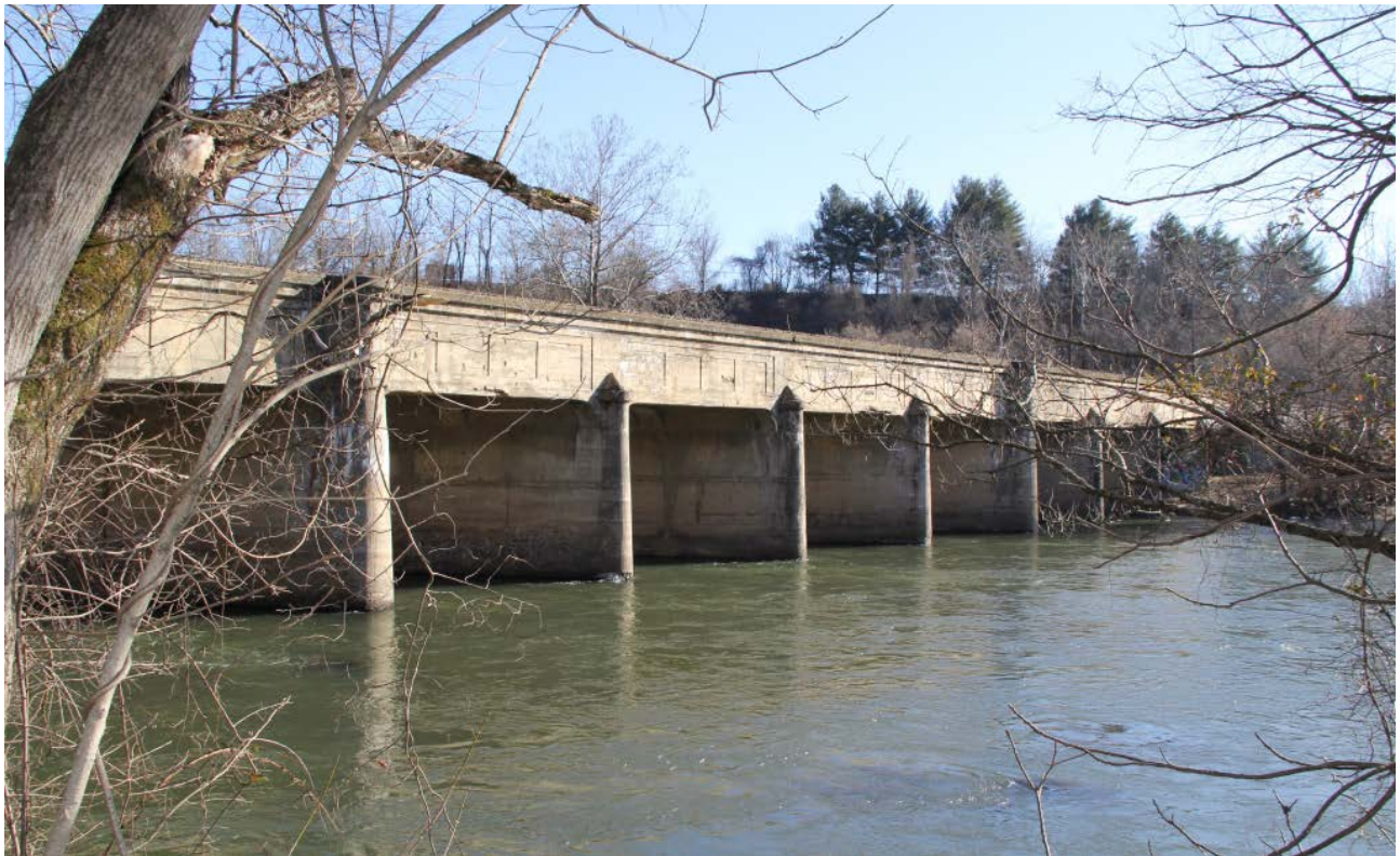
Southern Railroad Bridge over French Broad River, view northeast from Emma Road
